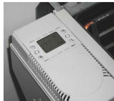
DISPLAY CONSOLE INSTALLED ON A FAN COIL UNIT
